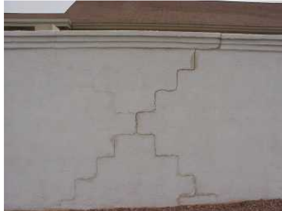
Damage associated with subsidence at 71st and Olive Avenues
